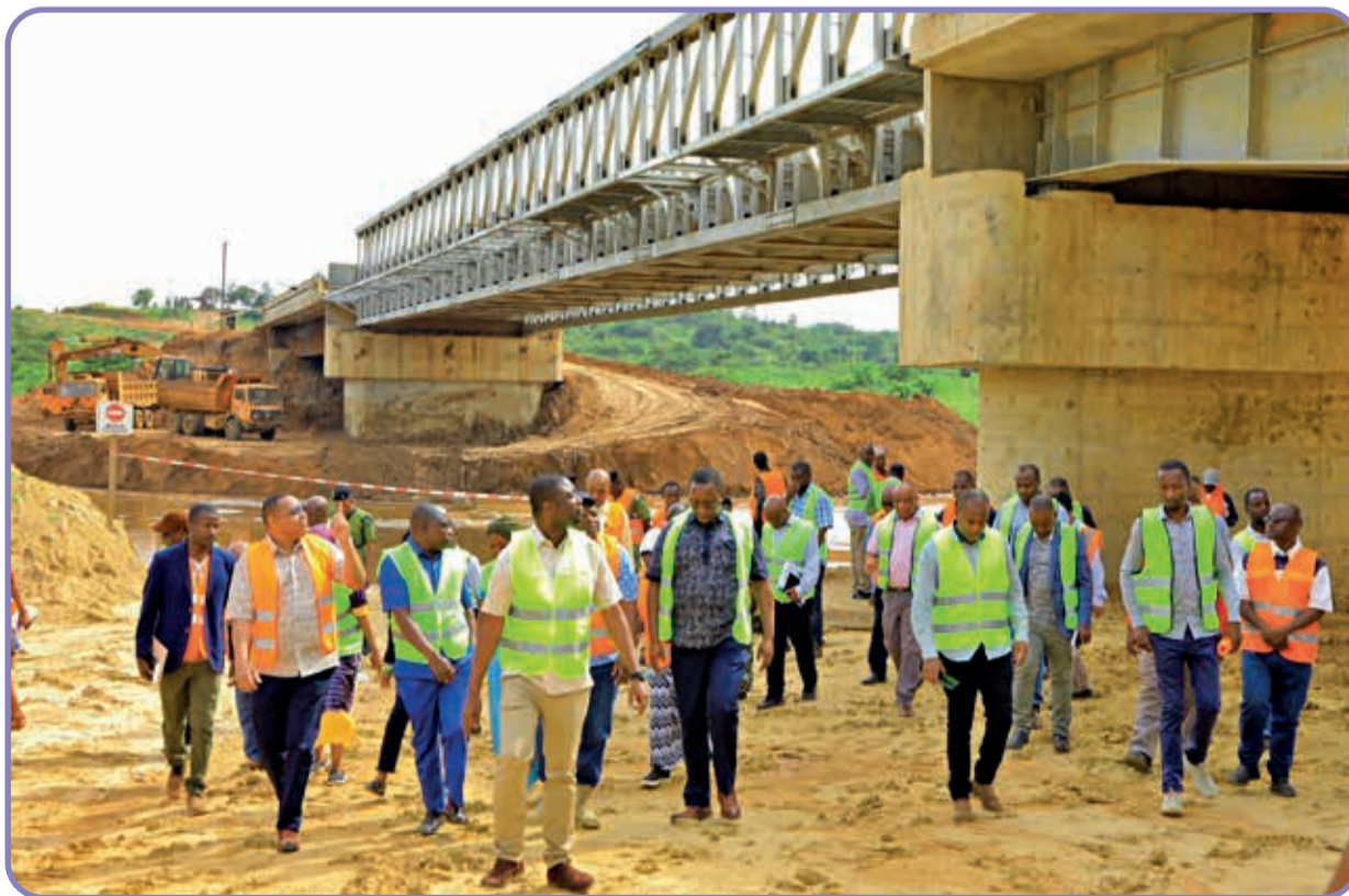
Members of the Parliamentary Committee on Infrastructure inspect construction of the 140m Kitengule Bridge. Construction of the bridge is being undertaken together with that of an 18-kilometre road linking Kyaka-Bugene-Benako and Kagera Sugar Junction-Kakunyu roads in Misenyi, Karagwe na Ngora districts in Kagera Region
